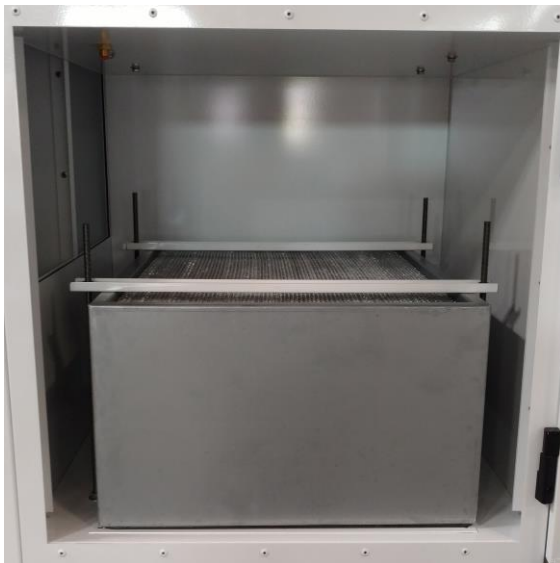
Figure 6: HEPA filter shown installed
