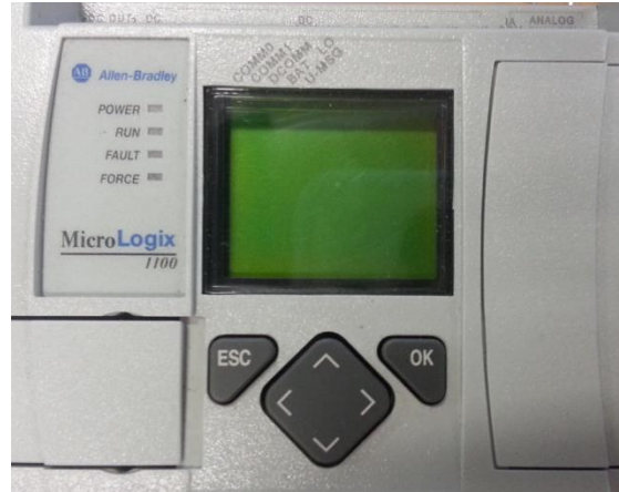
Figure 8: Internal PLC Panel
