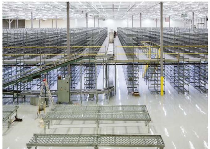
Multi-level system using E-Series Widespan shelving customized for conveyors in a distribution center with uneven floors.
